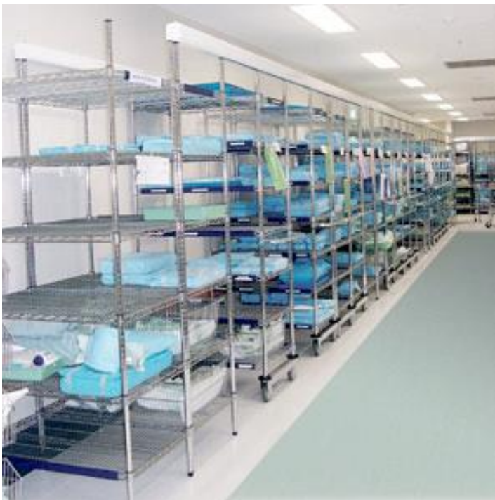
Figure 10: no sinks or hand basins in sterile stock storage areas
