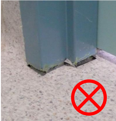
Figure 28: Gaps between door frame and floor
