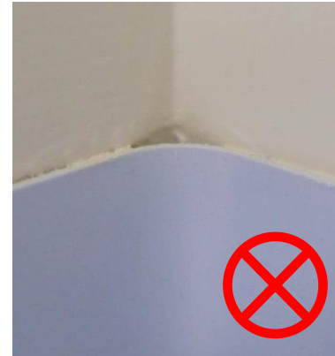
Figure 30: Gap between skirting and walls
