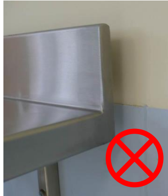
Figure 29: Gap between bench fitting and wall
